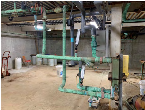
Current heat exchanger & downstairs pipe pictures
